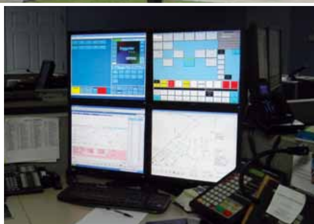
Top: The Tattnall County Judicial Annex in Reidsville, GA. Above: New display screens at Tattnall County 9-1-1.
