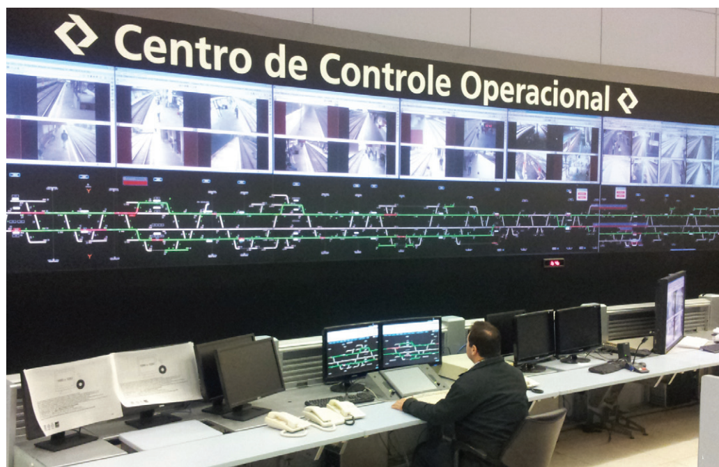
Zetron's Series 4000 is used to manage operations at CPTM's sophisticated communications control center.
