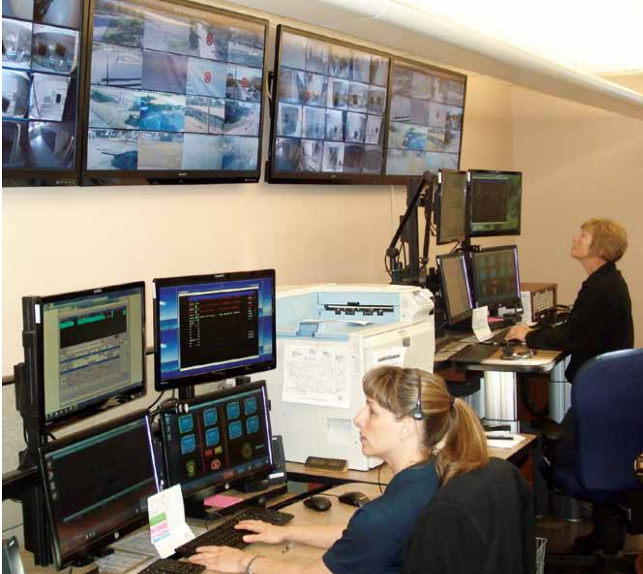
Dispatchers Anne Kluiber (foreground) and Yvette Kavouras utilize Lakewood's new MAX systems to handle their dispatching and 9-1-1 call-taking tasks.
